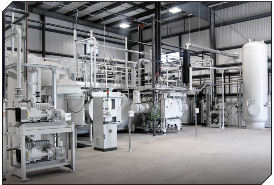
Modern high production low pressure carburizing furnaces at Nitrex HTS – Aurora, IL.
